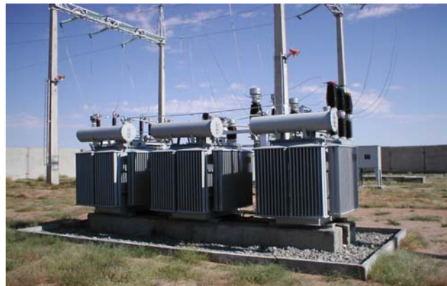
MCR 3.63 Mvar, 11 kV, Mongolia
