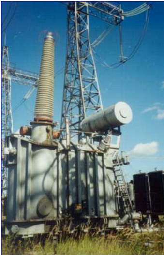
A phase of MCR-T type RODCU-60/525/ \sqrt{3} installed at Bely Rast substation, Moscow Region, Russian Federation
