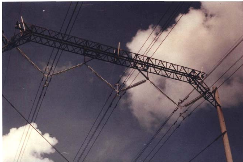
Fig.7. Compact 330kV line of 150 km with 4 subconductors, 1990 (Russia).
