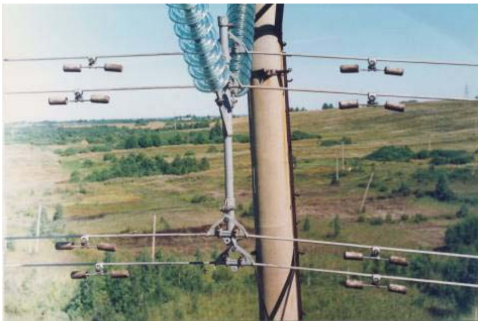
b) V-insulator set
